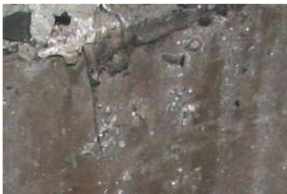
High energy splatter due to arcing*
