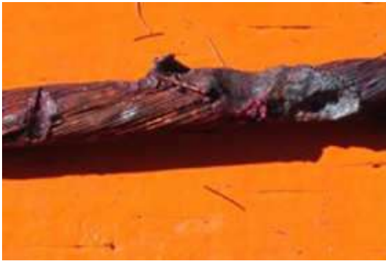
Arcing evidence: notching*
